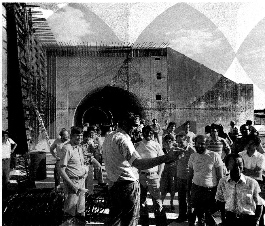
Participants at the Workshop had the chance to see the construction progress for the ISABELLE ring and experimental areas.
